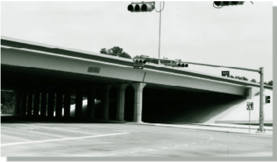
HPC is used in the superstructure and substructure of the Louetta Road Overpass in Houston, Texas.
