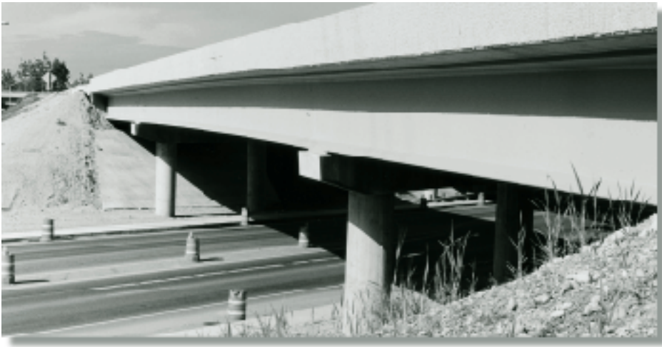
HPC was used in the girders and deck of Washington State HPC showcase bridge.
