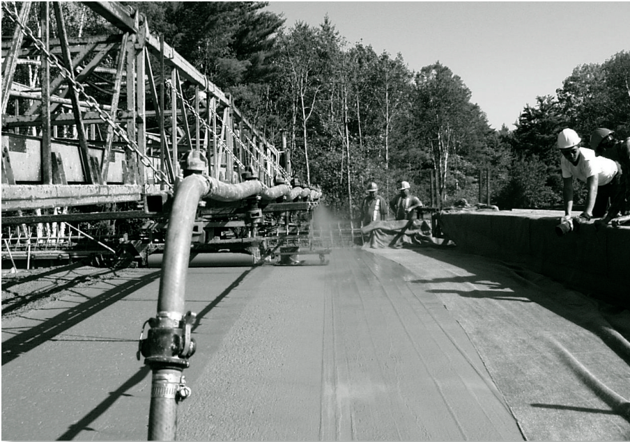
Application of wet burlap within 6-1/2 to 13 ft (2 to 4 m) of finishing equipment.
