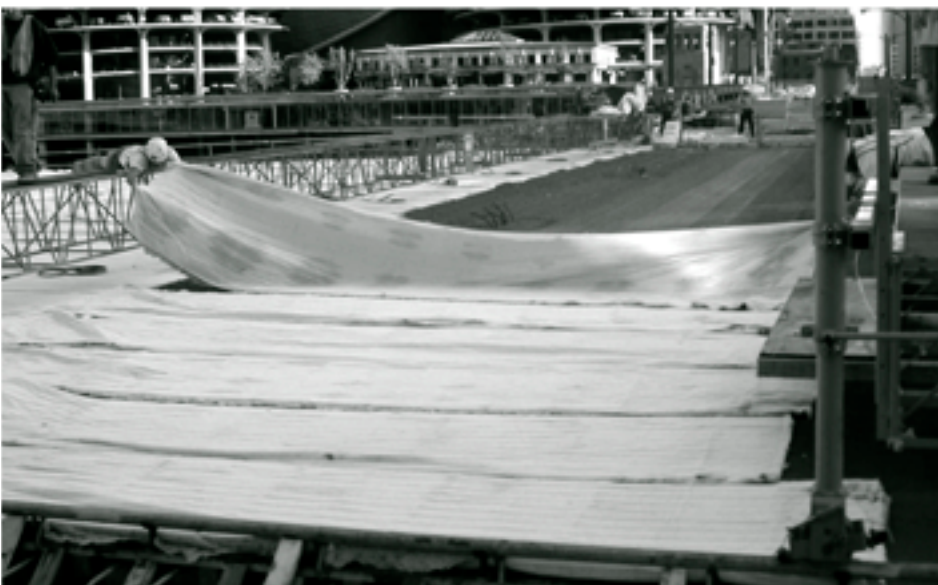
The surface of the concrete was required to be covered immediately after plastic texturing.
