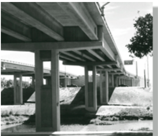
Fly ash was used in the San Angelo HPC bridge girders to enhance strength. (Photograph Courtesy of TXDOT)
