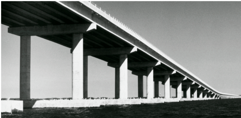
Concrete mix proportions were selected to provide a target service life of 100 years.
