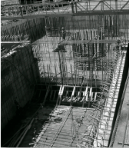
Cementitious materials in the tower footing concrete included 35 percent fly ash to minimize the heat of hydration.
