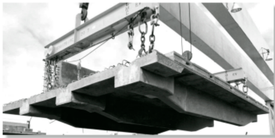
High performance concrete deck panels were used for rapid bridge deck construction.
