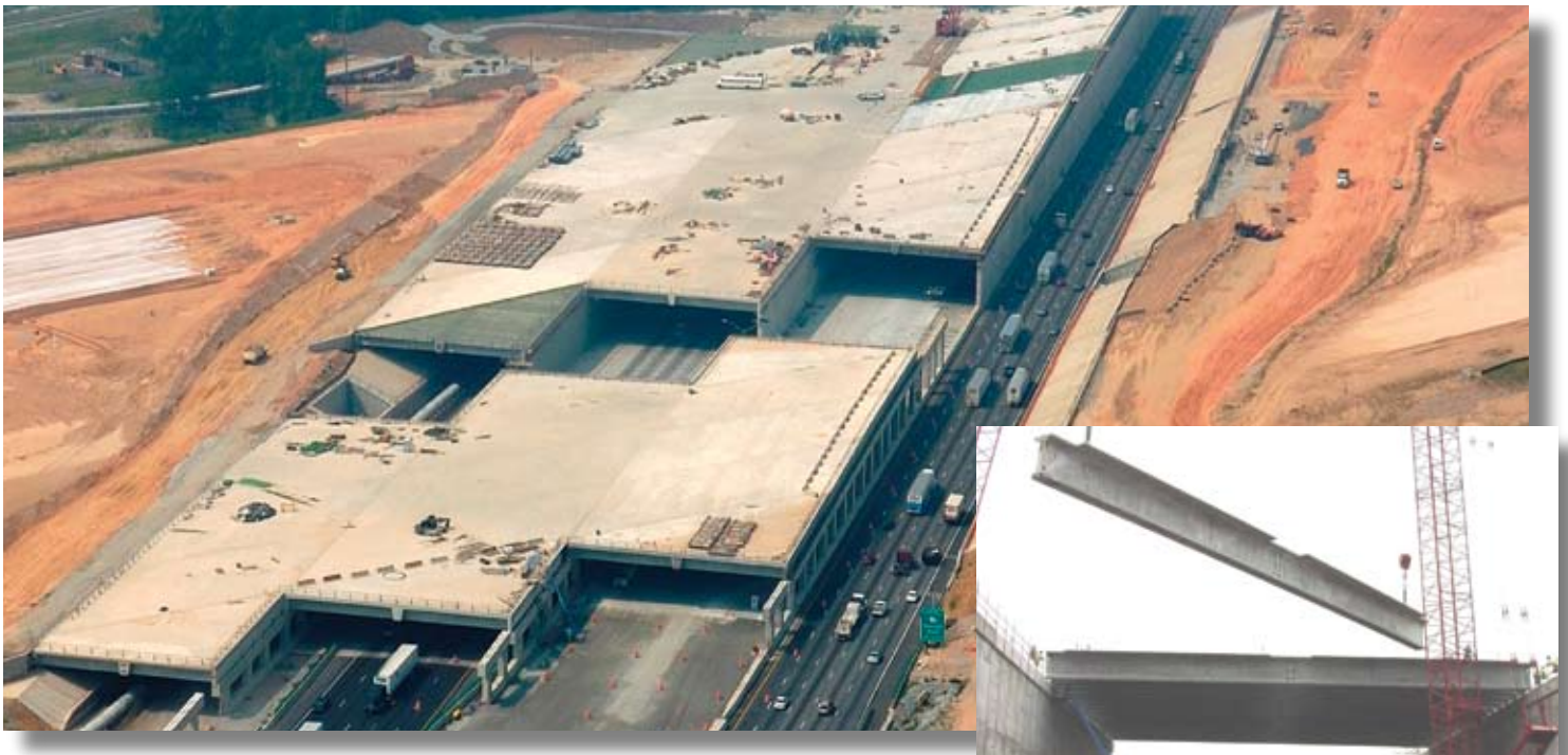
High-strength concrete was used in the precast, prestressed concrete beams across the interstate.
