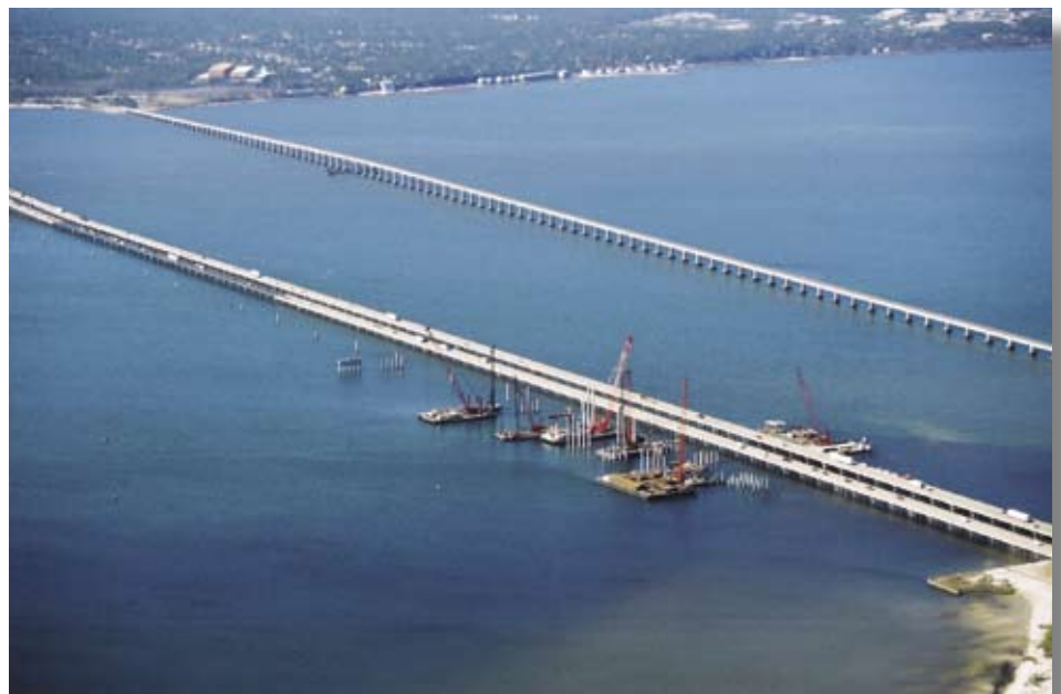
Construction of the new bridge alongside the existing bridge. Photo courtesy Parsons Brinckerhoff Construction Services.
