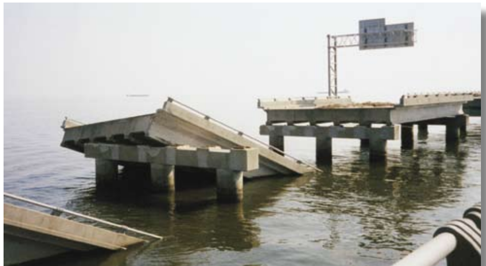
Collapsed spans on the I-10 bridge.
