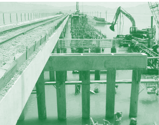
HPC was selected to achieve a 100-year service life in the salty environment.
