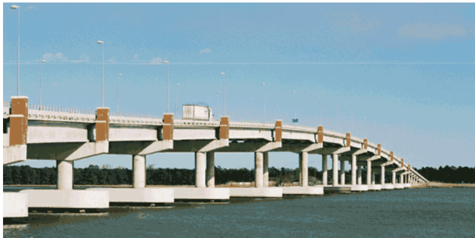
Lightweight concrete was used for the superstructure to achieve longer span lengths while reducing foundation loads.
