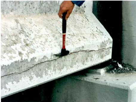
Crack induced in a prestressed concrete beam by alkali-silica reaction.
