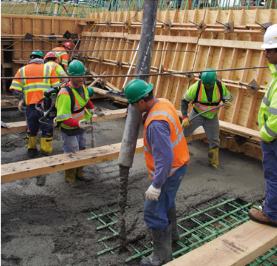
Casting the bottom flange of the cast-in-place superstructure. Photo: Tim Davis, FIGG
