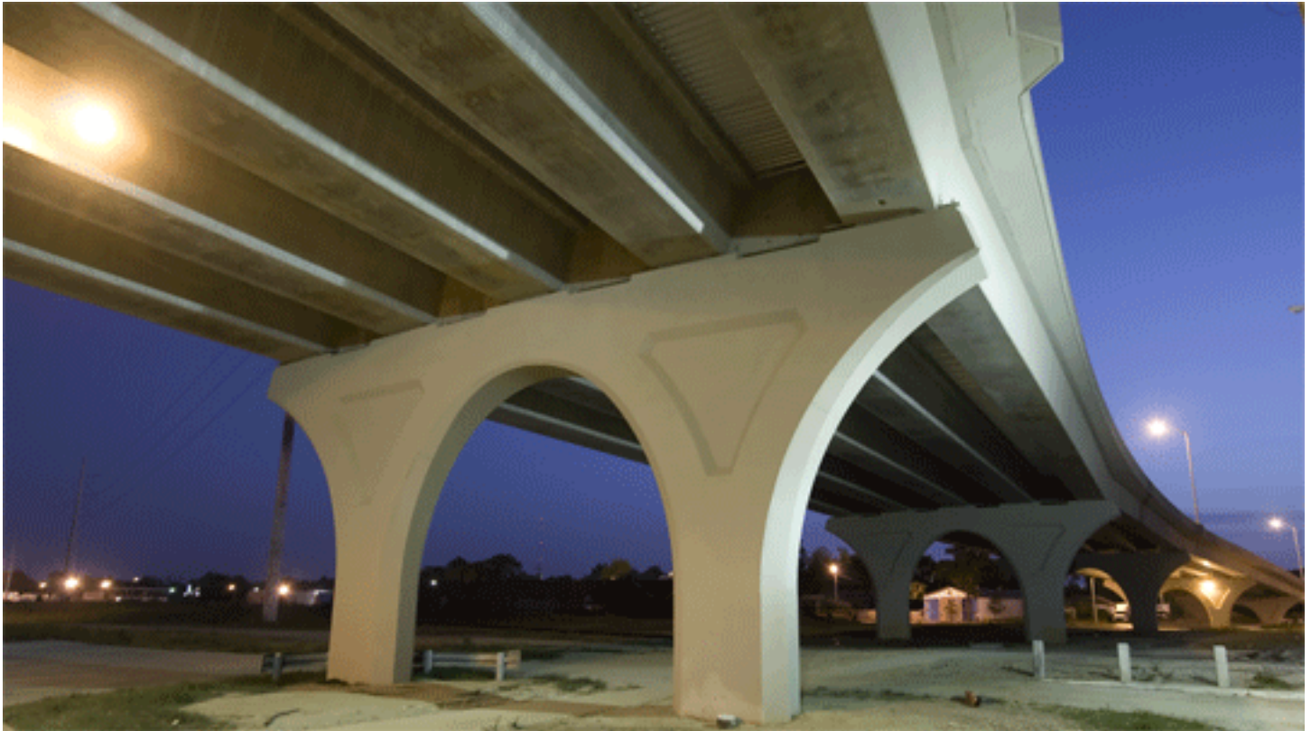
High strength concrete was used in the box beams to achieve a span-to-depth ratio of 29.
