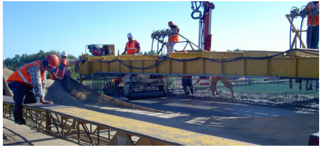
Wet burlap is placed within 10 minutes of strike-off for LC-HPC bridge decks.
