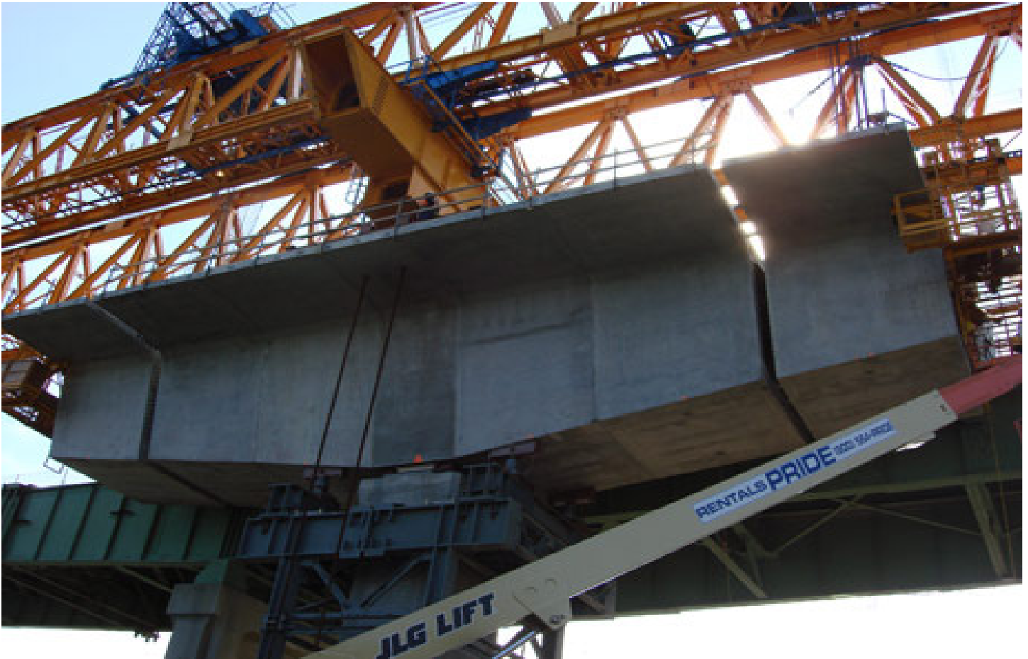
A concrete compressive strength of 10,000 psi (70 MPa) was specified for the precast superstructure and column segments.
