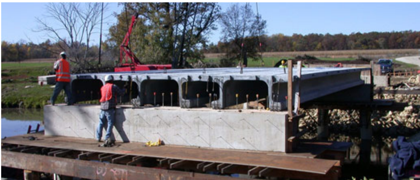
Ultra-high performance concrete was used in beams of the Jakway Park Bridge.
