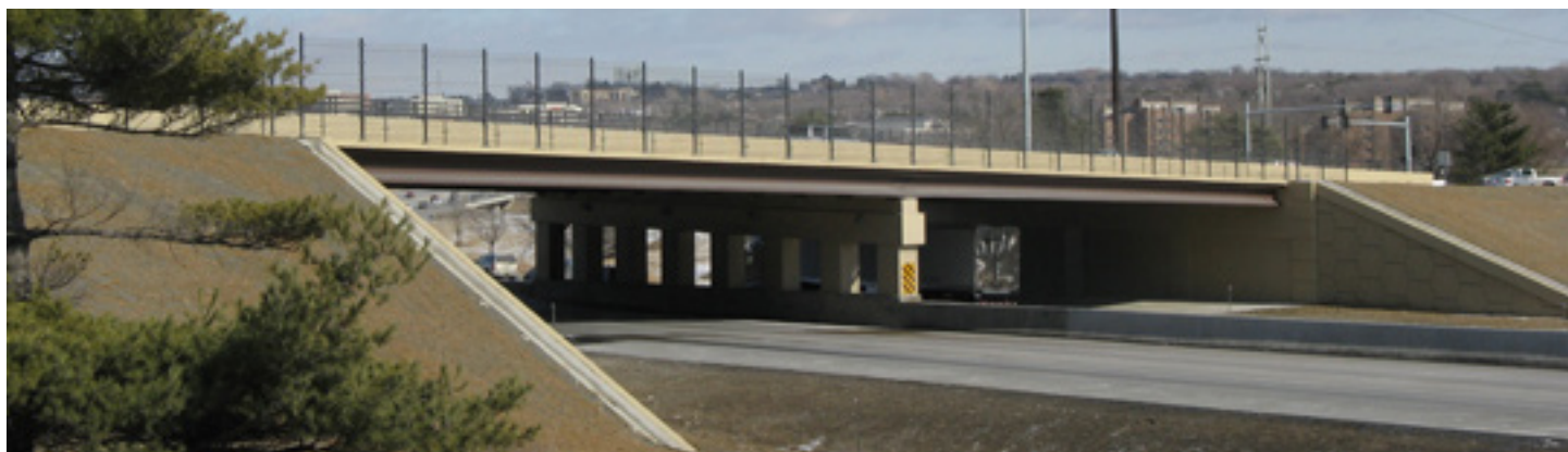
The Pacific Street Bridge, Omaha, NE, used 0.7-in. (17.8-mm) diameter strands in the precast, prestressed concrete beams.
