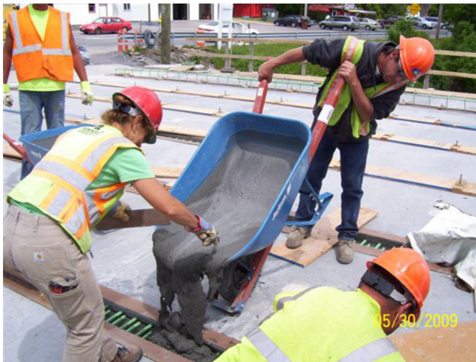
Placement of UHPC into the longitudinal connection between deck bulb-tee girders. (Photo courtesy of New York State DOT.)
