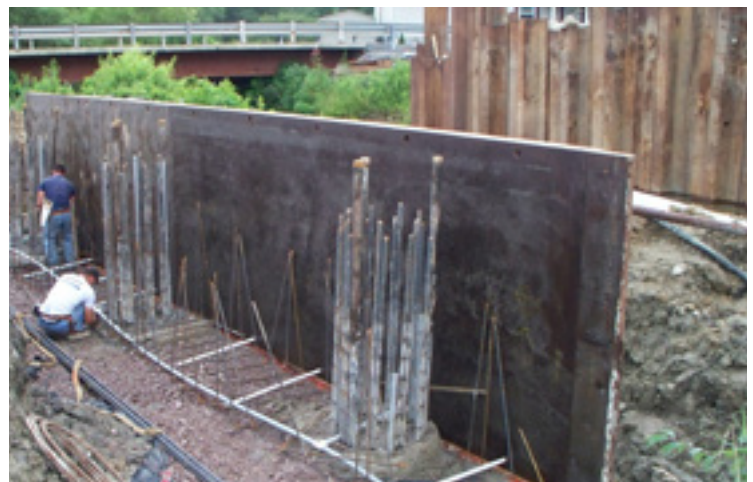
Reinforcement protruding from the tops of the three SCC caissons after completion.
