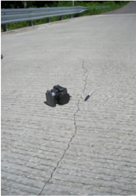
Fig. 2. Cracking that occurred when using a "conventional bridge deck mixture" in Monroe County, Indiana.
