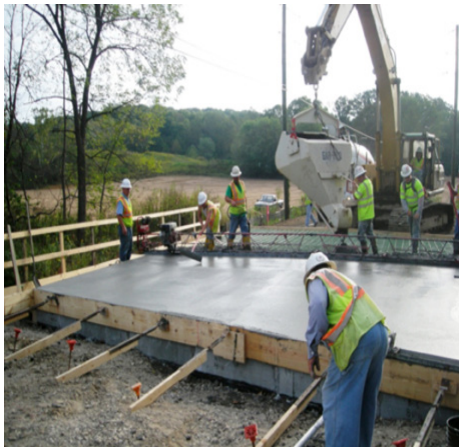
The photograph shows internally cured concrete being cast in a bridge deck Monroe County, Indiana.
