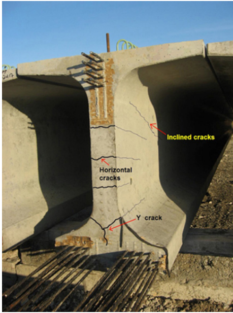
Fig. 1. An example of girder cracks
