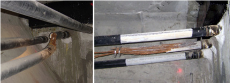
Fig. 3. Tendon failure in the Varina Enon Bridge because of strand corrosion.
