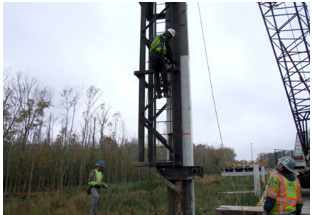
Fig. 1. Prestressed pile with Corrosion-Free Carbon Fiber Composite (CFCC) reinforcement being driven at the Nimmo Parkway Bridge site in Virginia Beach
