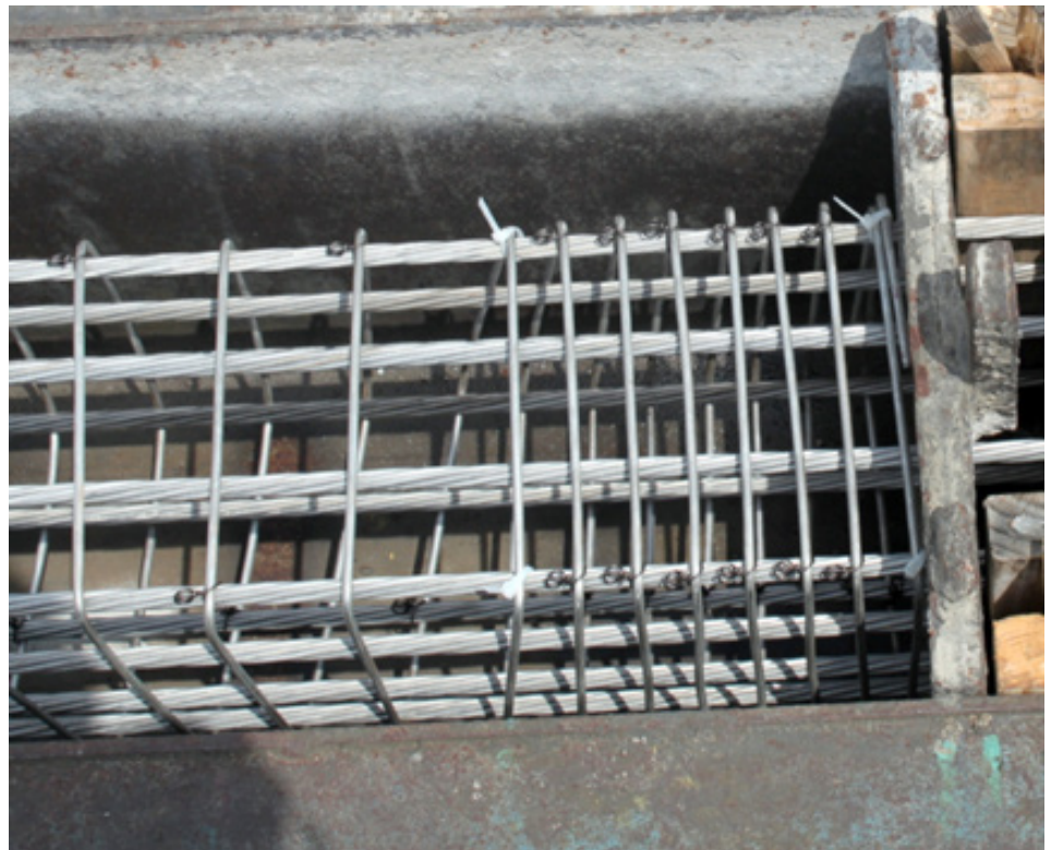
Fig. 1. 16-in. square pile with stainless steel grade 2205, 1/2-in. diameter 7-wire strands and with grade 304 stainless steel wire spiral.
