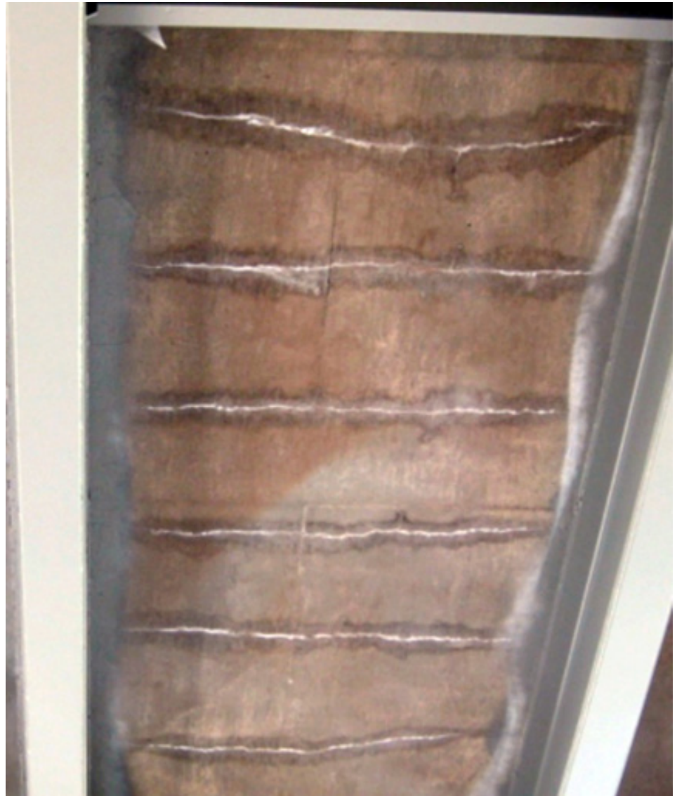
Fig. 2. Full depth leaking transverse cracks in concrete placed in a deck on I81 near Marion in 2009.
