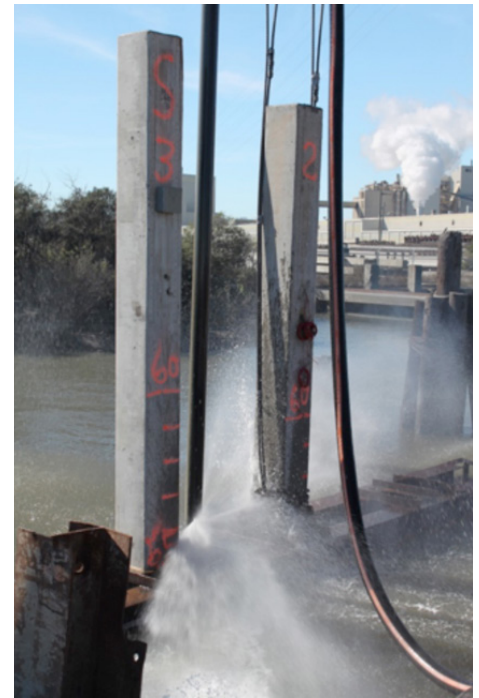
Fig. 2. 16-in., 70-ft long piles with stainless steel reinforcement being extracted after driving to refusal in Savannah River.
