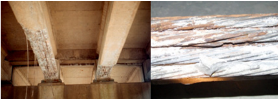
Fig. 2. Strands corroding in beams caused by leaking joints.
