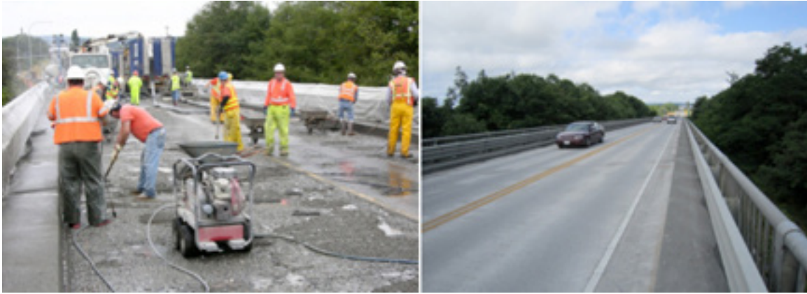
Fig. 1. The photo on the left shows SR532 near Stanwood, WA during construction.
