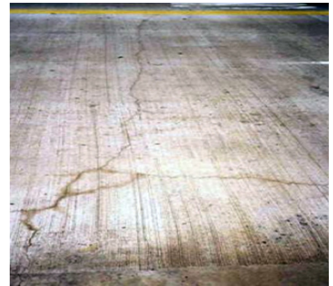
Fig. 4. Transverse Bridge Deck Cracking.
