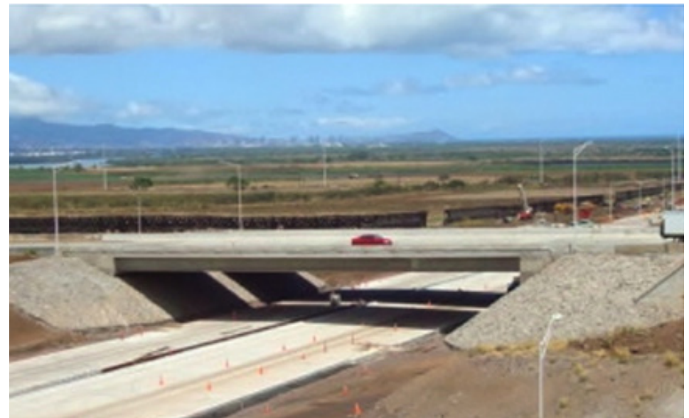
Fig. 1. Kualaka'i Parkway Grade Separation – No deck joints and No Shrinkage Cracks with use of SRA.
