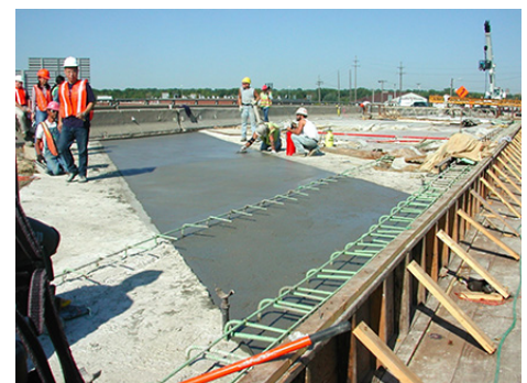
Fig. 1. Surface finishing of the ECC link-slab on the Grove Street Bridge in Michigan, 2005.
