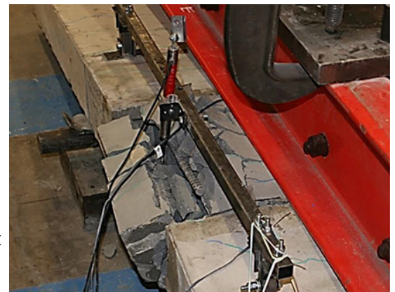
Fig. 1. Reinforcing bar-to-grout bond failure during fatigue loading in lab experiments carried out at Federal Highway Administration's Turner Fairbanks Research Center.
